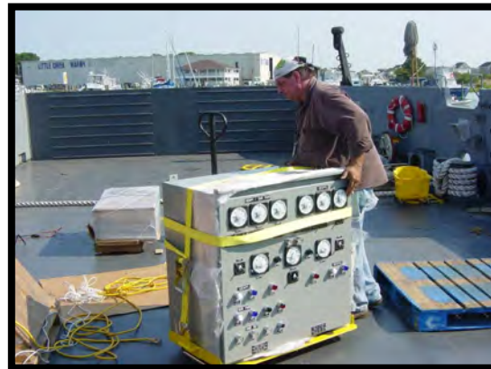
LCU Class SWBD Design and Installation
